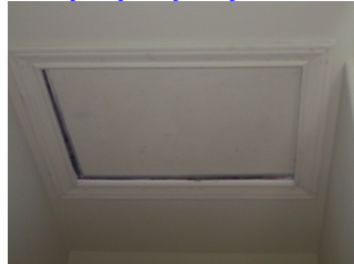
Excessive gap present at hatch
